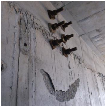
Structural cracks in wall W8A (Steel Bracket 'D' on the other face)
