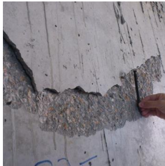
Close-up view of the structural cracks
