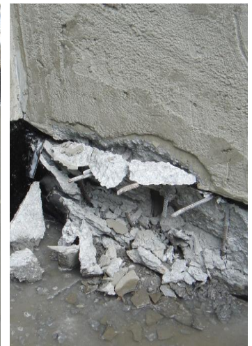
Shearing of rebars owing to pull-out failure of anchors
