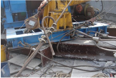
Steel base frame of hoisting crane (blue in colour) on spreader beams
