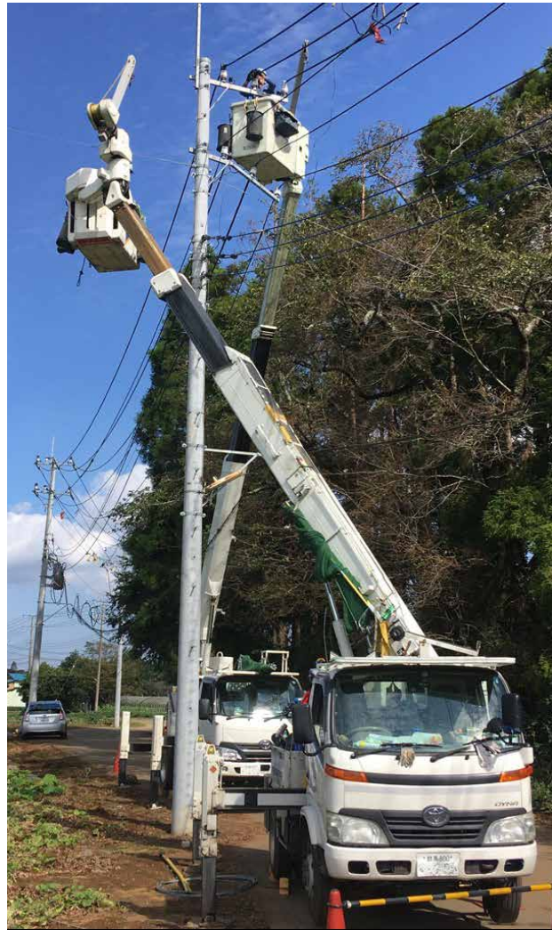
Photo courtesy TEPCO Power Grid
